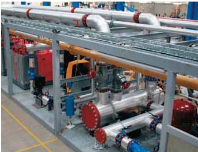
prefabricated M&E for the NHS
