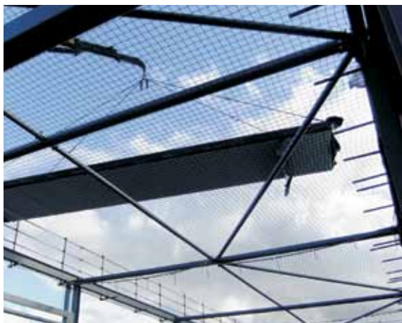
A 12.5m long SkanDek element being placed on the Heathrow snow blower storage building
