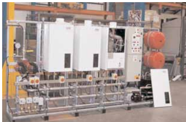
courtesy Armstrong Integrated Systems Limited
